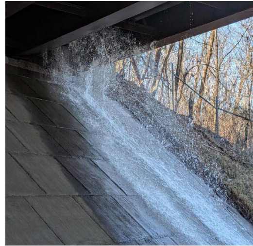
12-inch watermain break from west side abutment under Brandon Avenue Bridge over Rte. 220/I-581
