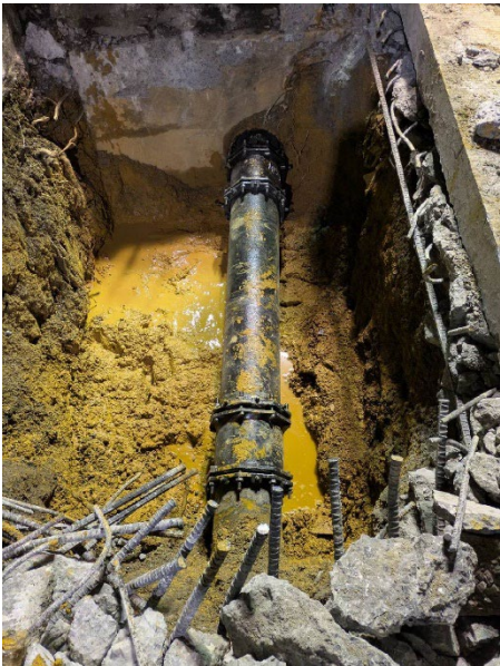
Replaced portion of 12-inch ductile-iron pipe under approach slab and through bridge abutment
