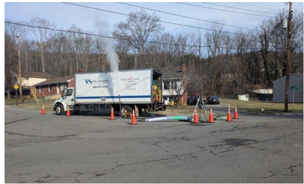
Visu-Sewer set up at a manhole installing a cured-in-place liner in the sewer main
