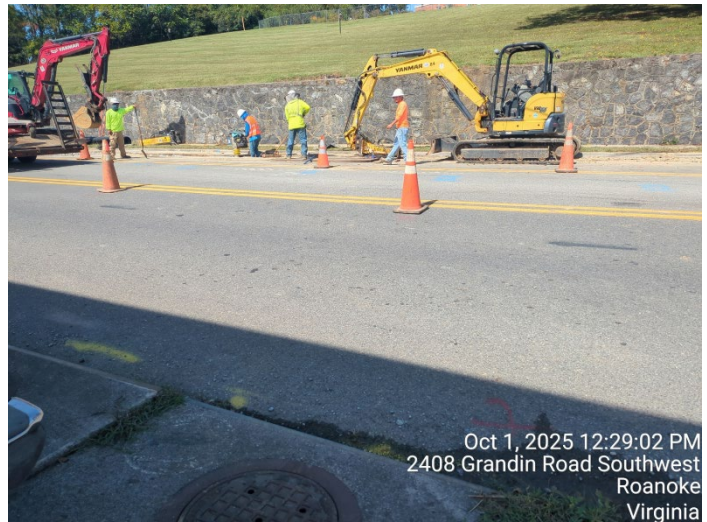
Grandin Avenue Waterline Replacement Project – Phase 2 (from Guilford Avenue to Beverly Boulevard)
