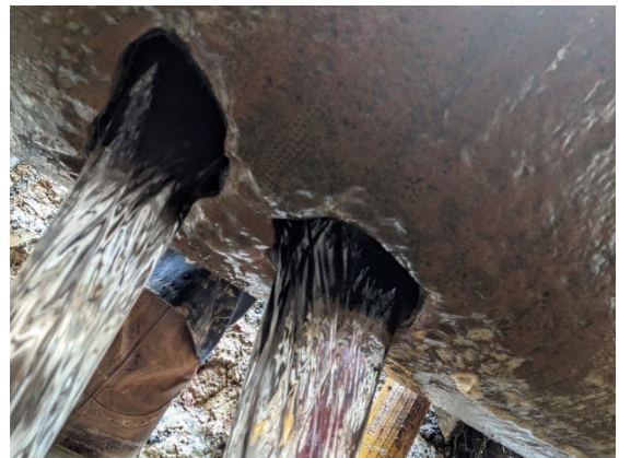
Two holes in the pipe were found to be the cause of the 16-inch water main break on Peters Creek Road
