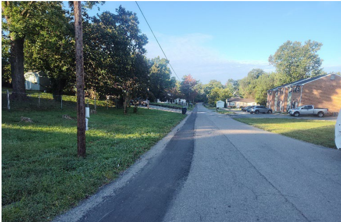
Base paving completed on a portion of the Eastgate Avenue Waterline Replacement Project prior to the City milling and overlaying
