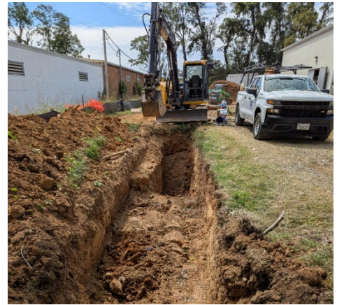
Statesman Pump Station Interim Improvements and Pipe Installation for tie-in to existing 20-inch Watermain
