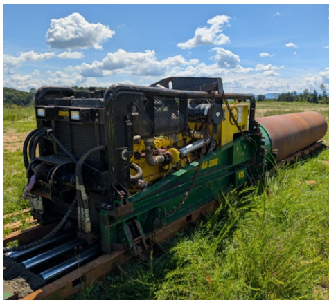
Boring Machine with Auger and Cutting Head Assembly for the Wood Haven Technology Park Waterline Extension Project
